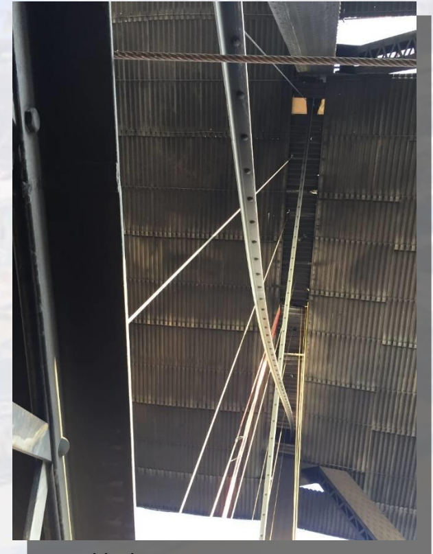
Buckled Sway Bracing near Pier 7
