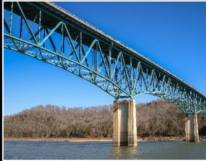
Hurricane Bridge Rehabilitation (SR 56) over Center Hill Lake, DeKalb County, TN Modjeski and Masters, Inc.
