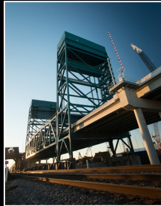
Henry G. Gilmerton Bridge over the Elizabeth River Modjeski and Masters, Inc.
