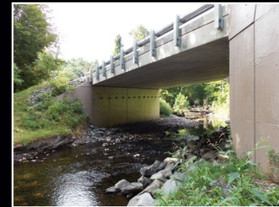
US 209, Raymondskill Creek Bridge, Delaware Water Gap National Recreation Area Johnson, Mirmiran & Thompson, Inc.
